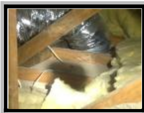
mis laid insulation
