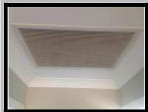
return air vent
