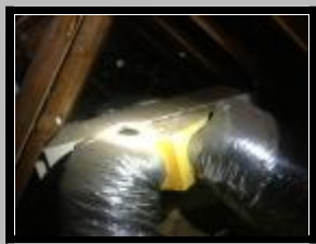
air conditioning blocking access
