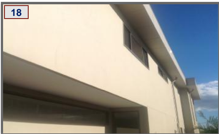
Right Hand Side - Exposed sheet joints to 2nd level
