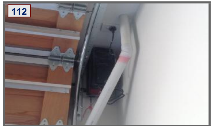
PVC pipe not secure
