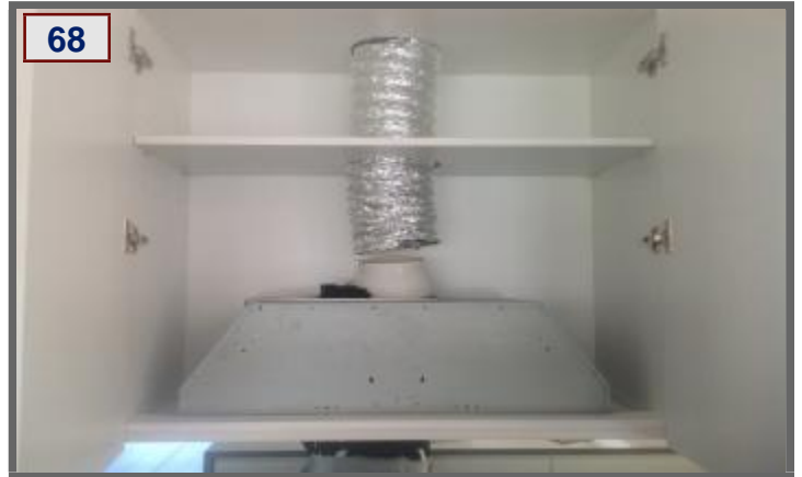
Rangehood duct not connected
