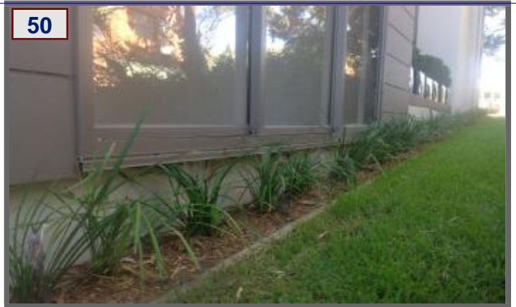
Not support under window
