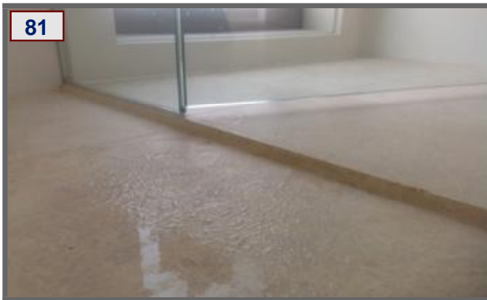
No exposed water stop
