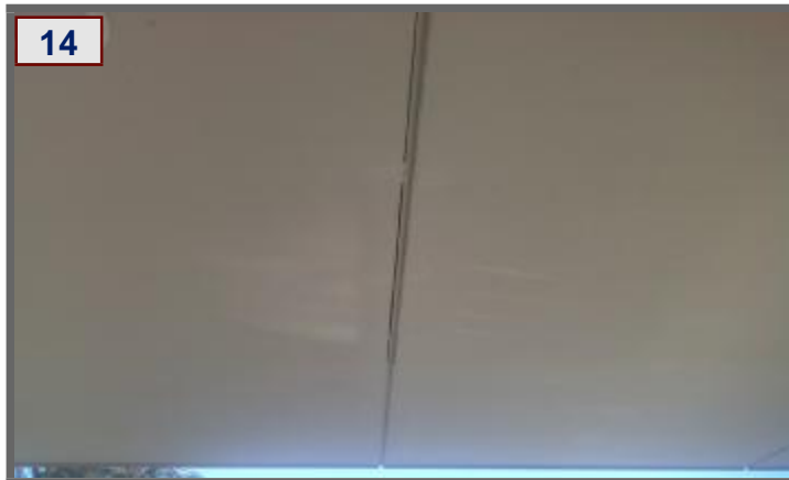
Cracking to soffit lining of Rear left Bedroom Balcony
