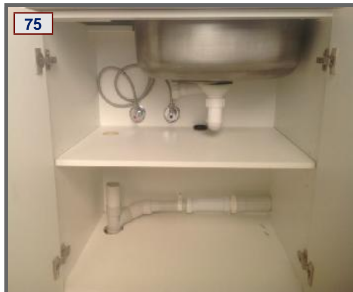
Laundry tub not waste not connected
