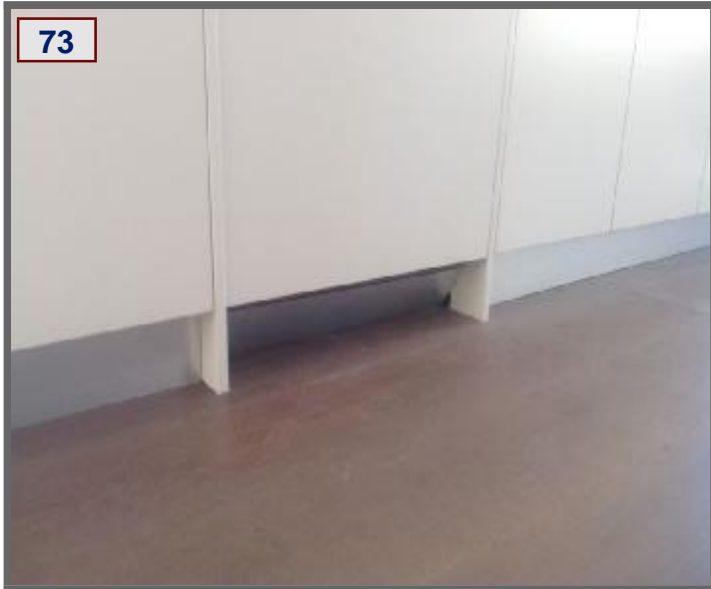
Kick panel under dishwasher not secured
