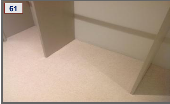
Skirting Missing to Bed 1 WIR
