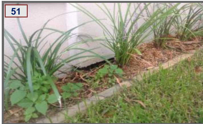
Blue Board in contact with the ground
