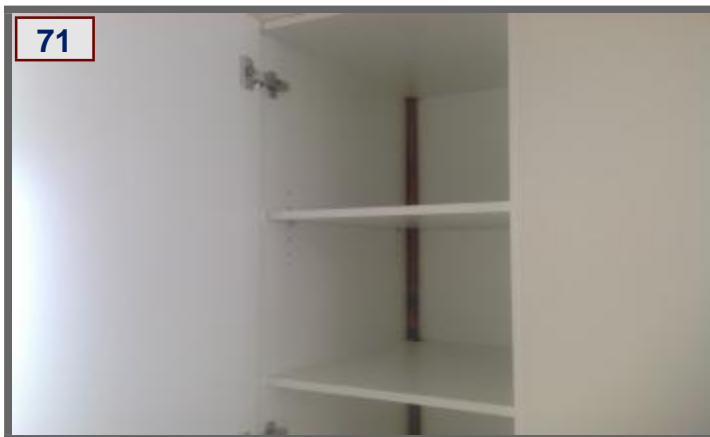
Exposed copper gas pipe
