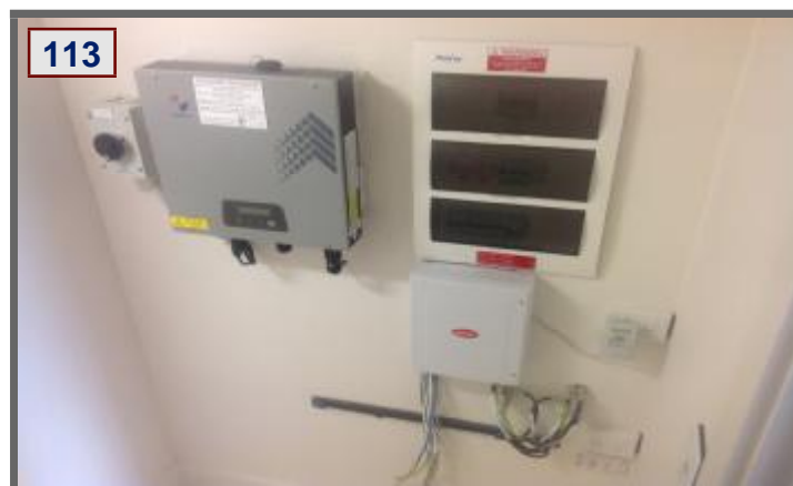
Electrical Sub Board in adjacent room
