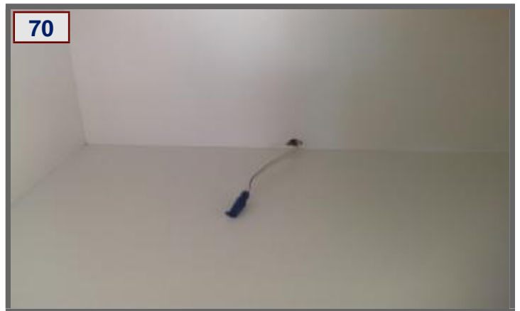
Exposed electrical wire
