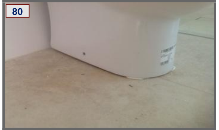
Toilet not secure
